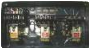
Interior View of MK1 SASD
