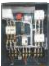
Interior View of MU-G30W FASD
