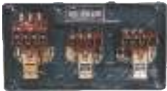
Interior View of MK2 SASD
