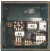
Interior View of MU-G20W FASD
